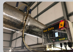
Gas Flow Monitoring
